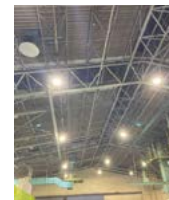
Interior LED lighting
